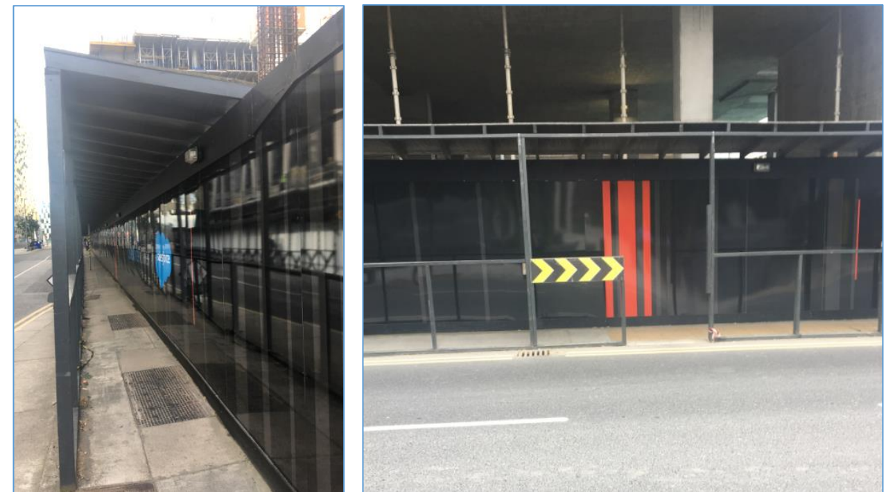
Covered Walkway at RGRE Spencer Place South Construction Site – Same Robust and Well Maintained Type of Walkway & Hoarding to be used on this Project
