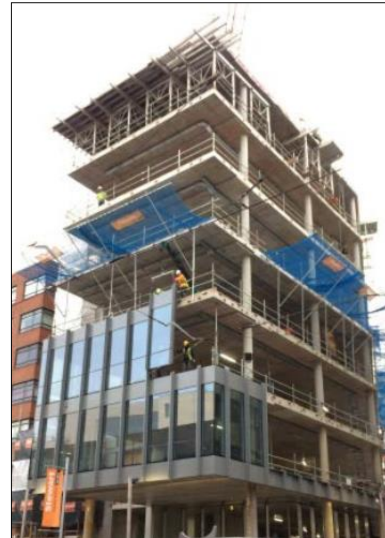
Unitised Façade Installation – Mini Crane on Floor Above Lifting Unit into Position; Debris Net Fans Above.
